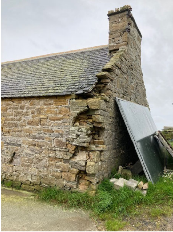
Damaged corner to bothy.
