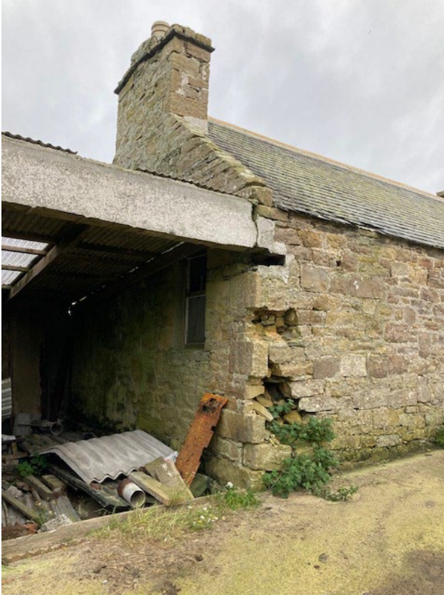
Damaged corner and lean-to-shed at bothy.
