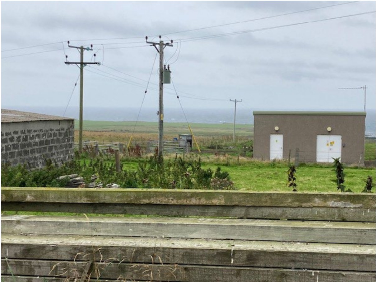
Electric Substation and overhead cables
