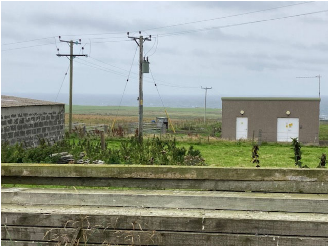
Electric Substation and overhead cables
