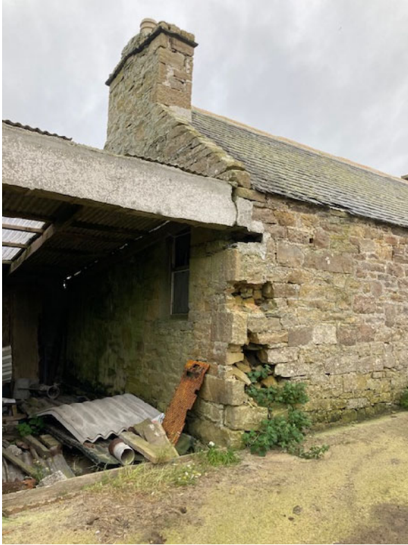
Damaged corner and lean-to-shed at bothy.
