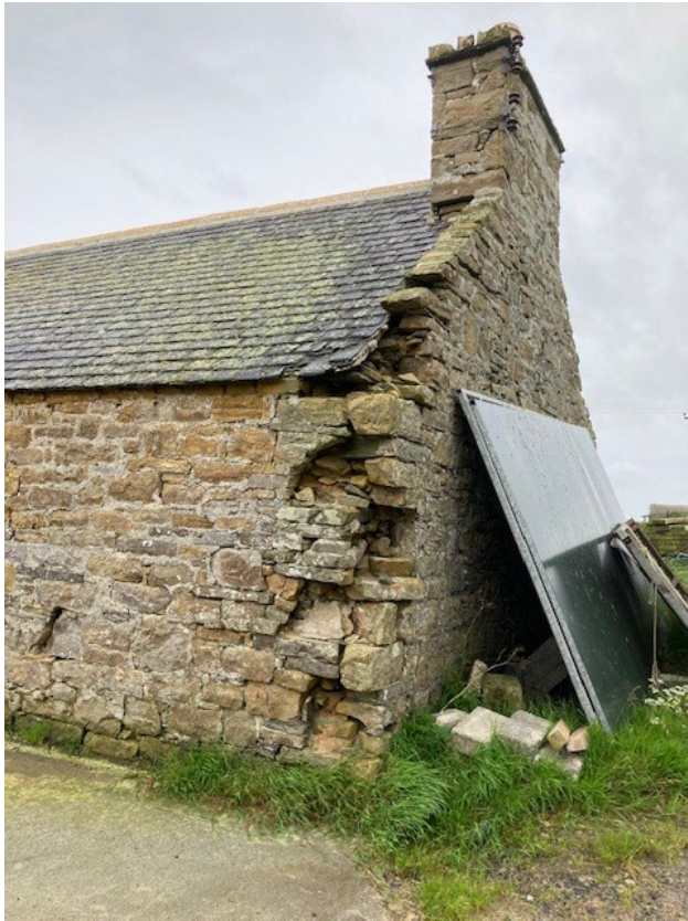
Damaged corner to bothy.
